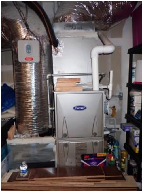
The furnace appeared serviceable
