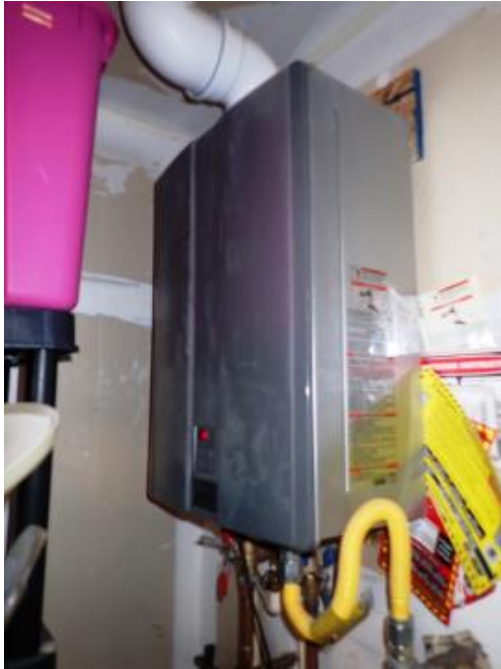
Tankless water heater located front right corner of garage
