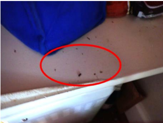
There appears to be mouse droppings on one of the pantry shelves on the right
