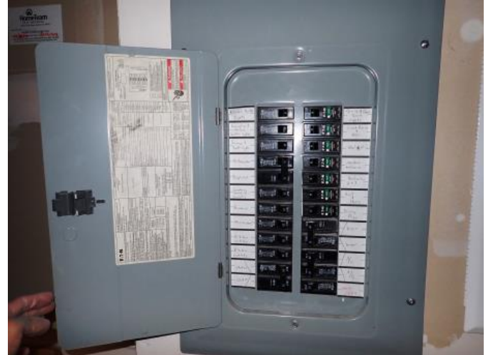
All breakers appeared serviceable with labels
