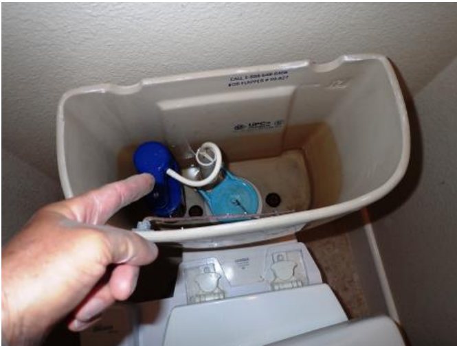
The primary bathroom toilet did not refill when flushed. Needs further evaluation
