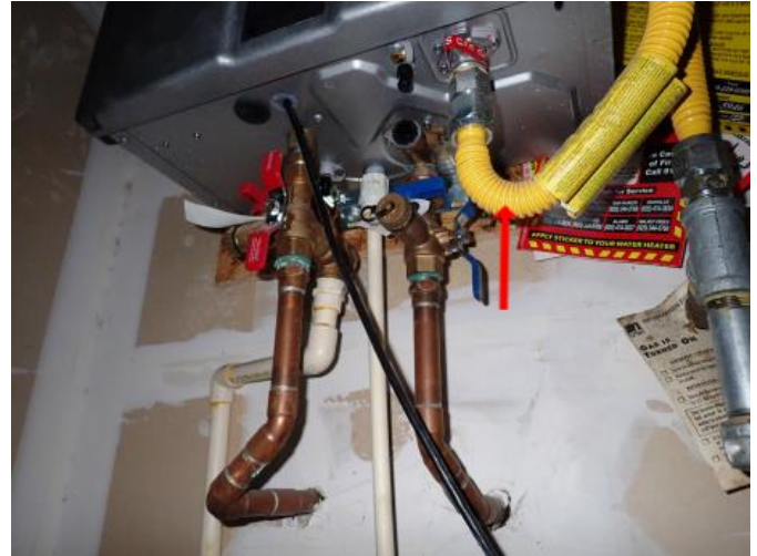
All water and gas shut offs are located below the unit. Gas shut off is the yellow line
