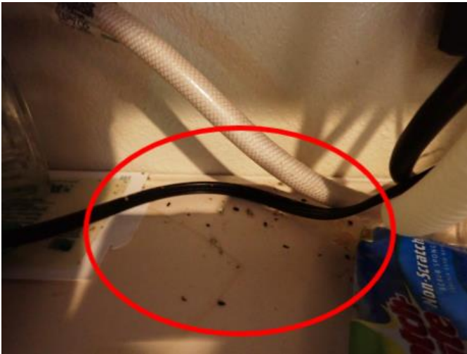
There appears to be mouse droppings under the kitchen sink cabinet
