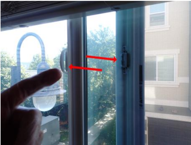
The back dining room window does not latch when closed
