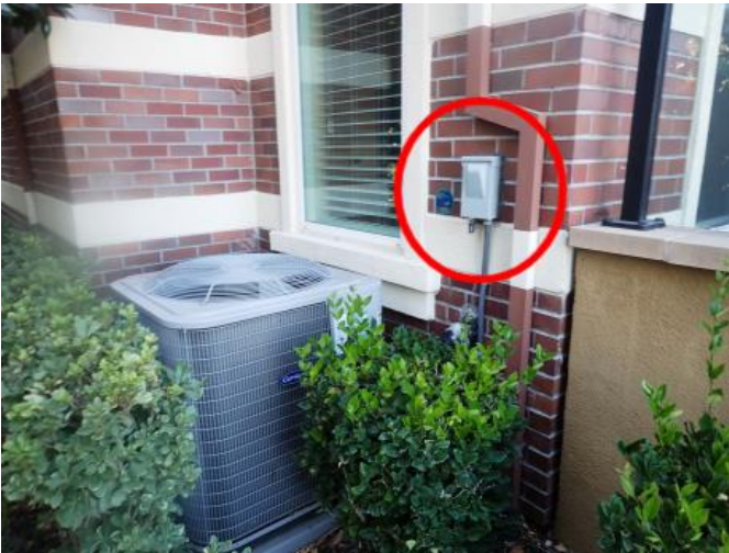
AC unit front left exterior of the townhome. Master shut off on wall behind
